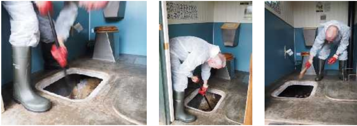
Raking the compost towards the door end and sweeping the flange before refitting the hatch.
