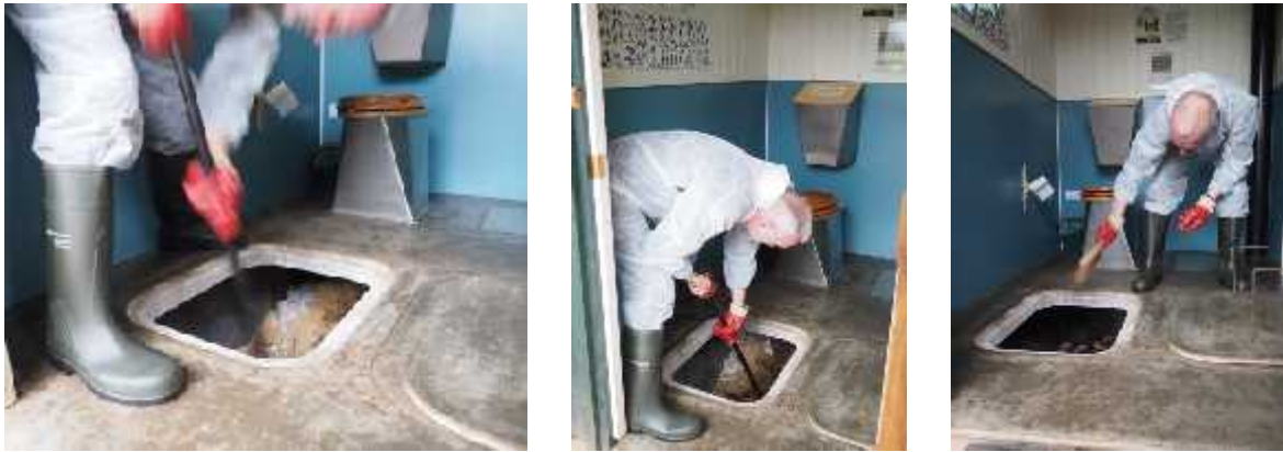
Raking the compost towards the door end and sweeping the flange before refitting the hatch.
