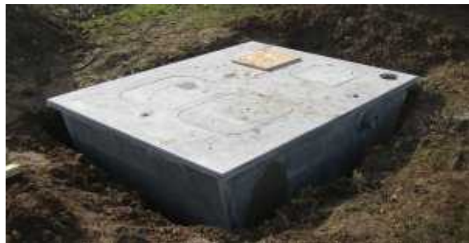
A view from the front RH corner of the building. The ventilation socket is in the back RH corner.
