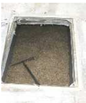
Rake rested inside active vault.
