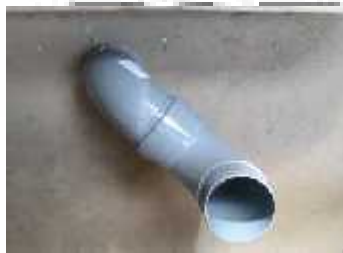
Vaults with grey S bend connected to urine outlet
