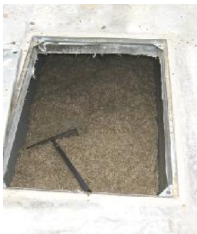
Rake rested inside active vault.
