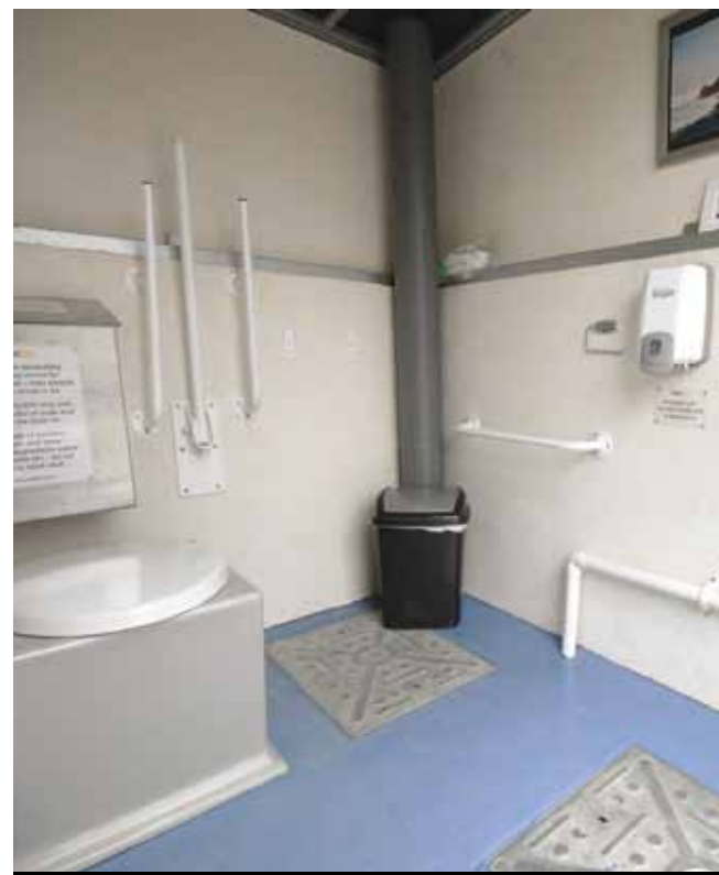
This compost toilet, in an allotment in Cardiff, was installed earlier this year and has since been decorated by the allotment group
