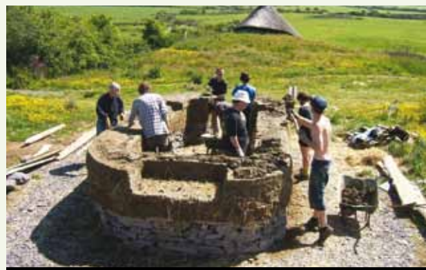
A new cob walled and thatched compost toilet being built at Menter Felin Uchaf, Wales
